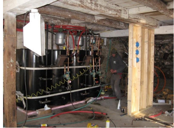
Initial system with tanks
