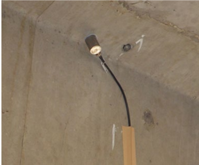
Figure 3.1: Acoustic emission sensor attached to a concrete girder (Figure courtesy Mistras Group)
