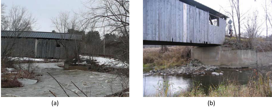
Figure 2.2: The view of the bridge from upstream during a high-flow event (a) and cracking and undermining of the abutment of the bridge due to scour (b).
